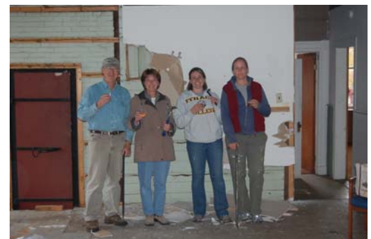
AARCH staff on day one—removing late 20th century alterations to the interior of the building. Note the vault (left) that was revealed behind a partition.
