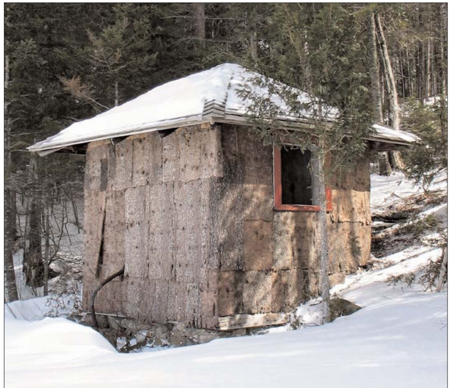
The Pump House, on Lake Newcomb, with its birch-bark siding recently restored.
